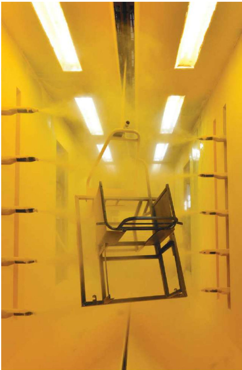
Automatic Powder Coating booth plant.
