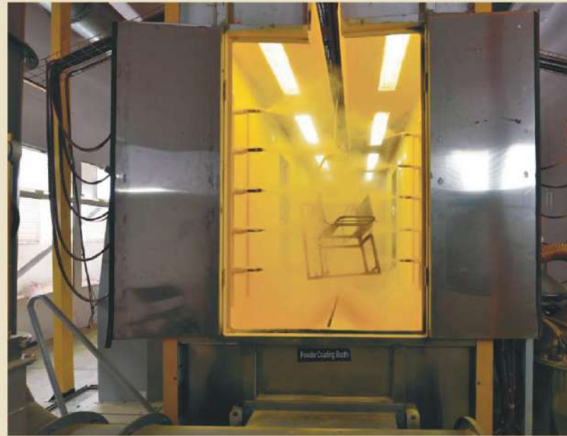
Powder coating booth at work center-6.
